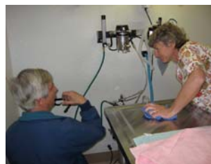
Jeff Lee to the rescue to fix leaky tank
